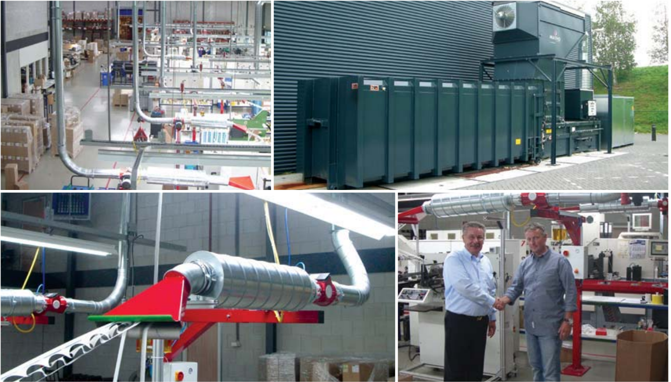
TOP LEFT: production environment with central pipe and a lot of EM-Modules (exhausting modules) for the extraction and cutting of edge trims and matrix TOP RIGHT: press container with air-material-separator, main ventilator and balance ventilator outside the plant. BOTTOM RIGHT: Josef Thor, Managing Director Matho GmbH; Right Jack Willemsz, Managing Director W&R etiketten shaking hands after finishing installation and acceptance of the system BOTTOM LEFT: EM-160 module on every label press, cuts the matrix and edge trim waste and extracts it through the main pipe to the press container outside.
